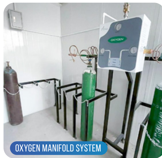
MEDICAL GAS ZONE VALVE AND ALARM SYSTEM
